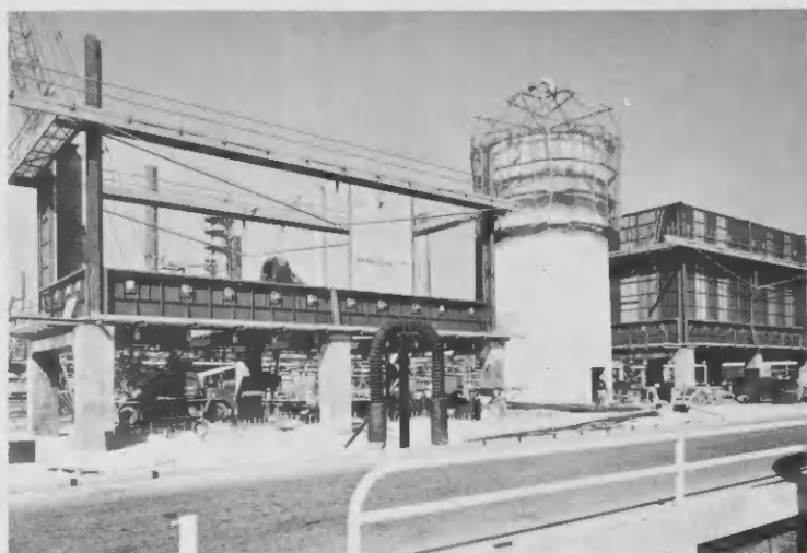
The two furnaces for Pipestills 5 & 6 rising near the north refinery road with a concrete smokestack in center that will be 350 ft. high and serve both furnaces.
